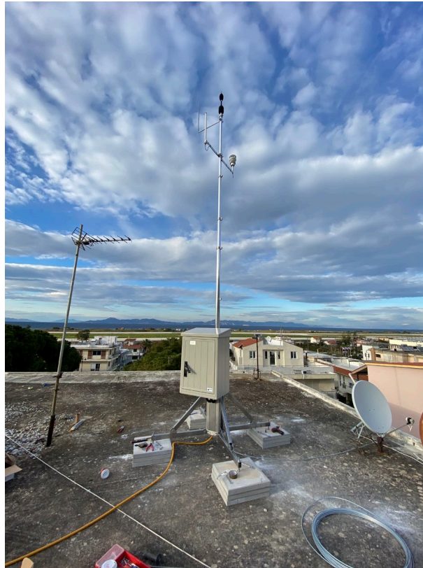
Figure 11 - Typical installation of Noise Compass in an unattended monitoring station.
